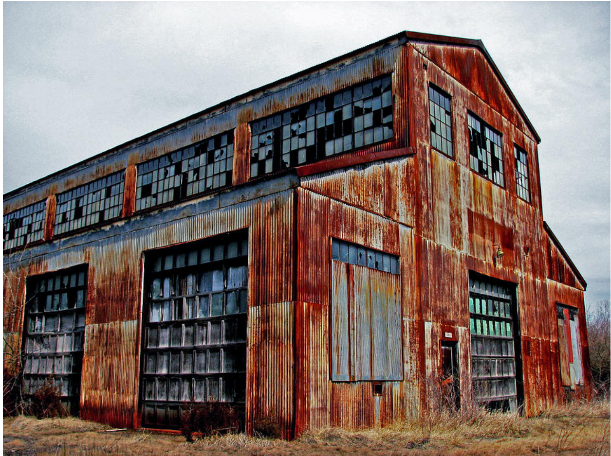
7 Warehouse exterior with busted windows [4]
